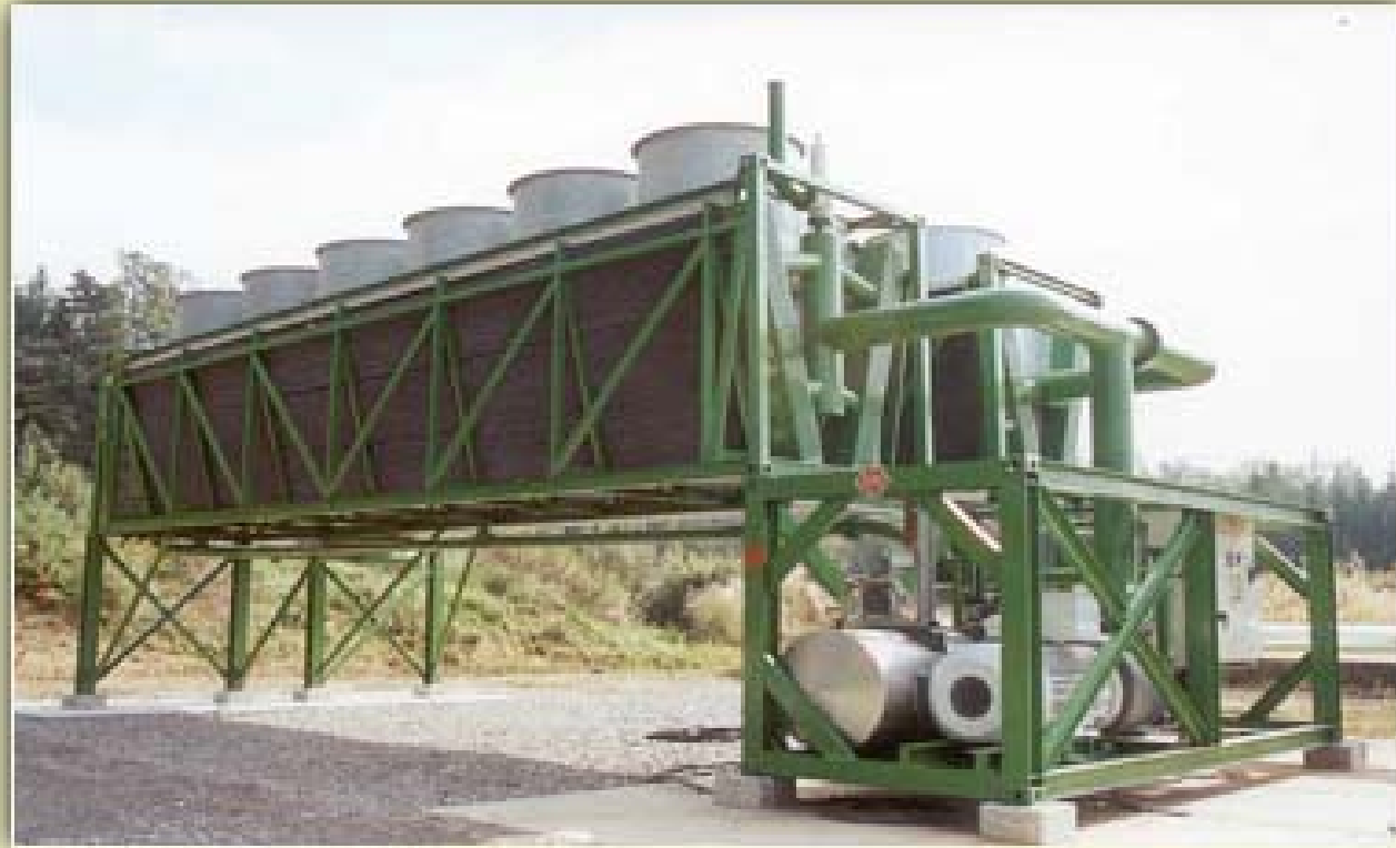
Ormat 250 kW air-cooled Geothermal CHP Plant
