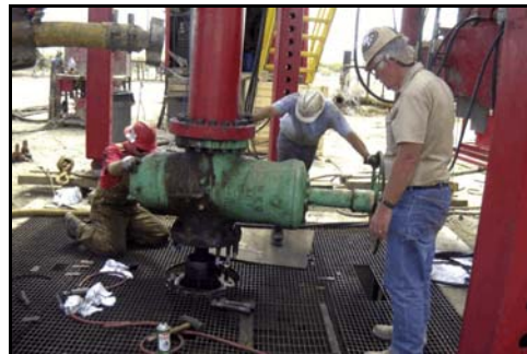
Drill rig workers during the well workover at Raft River, Idaho. (Photo: U.S. Geothermal Inc.)
